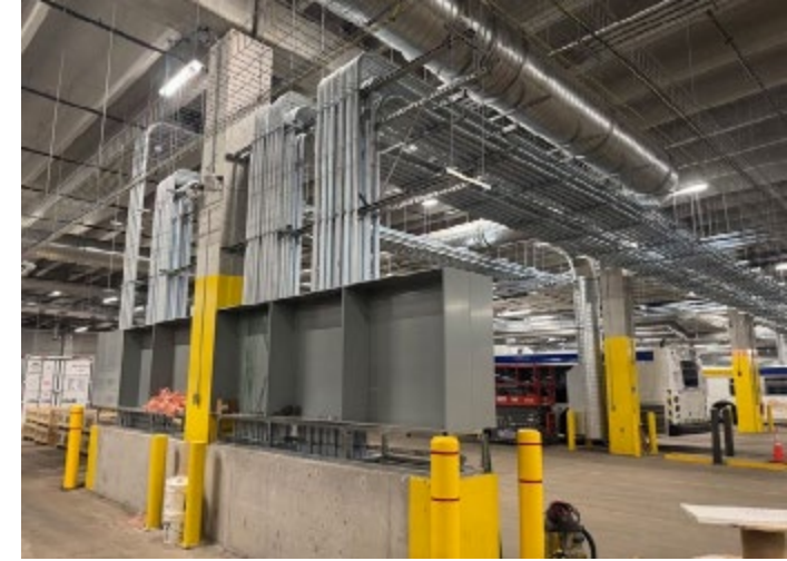
Garage Bus Chargers - Metro Transit North Loop; Minneapolis, MN
