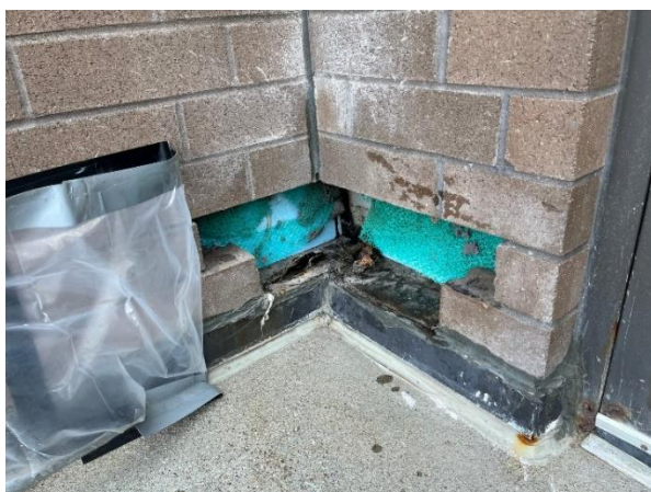
Figure 14: Destructive Test Opening 3 at inside corner adjacent to access door.
