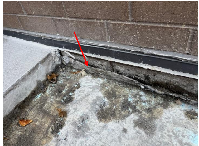
Figure 18: Plaza waterproofing de-bonded at base of wall.
