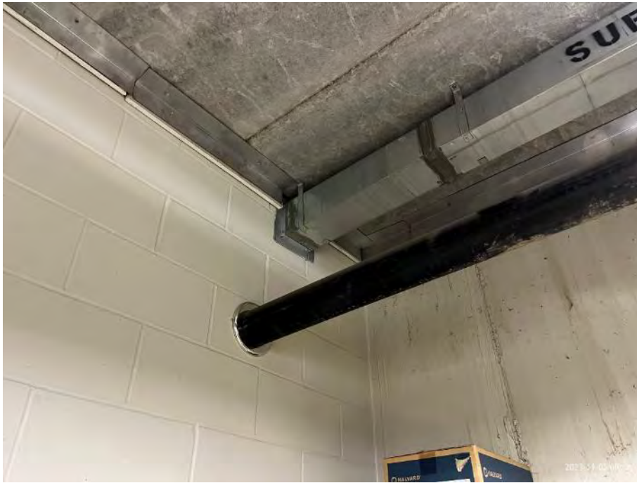
Photo 11 – Northeast corner of Patrol Equipment Room. Evidence of water staining from multiple reported leaks.
