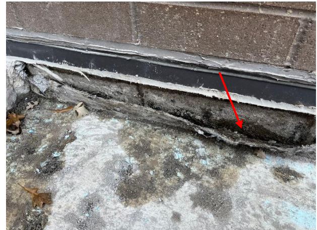
Figure 20: De-bonded waterproofing at CMU starter courses
