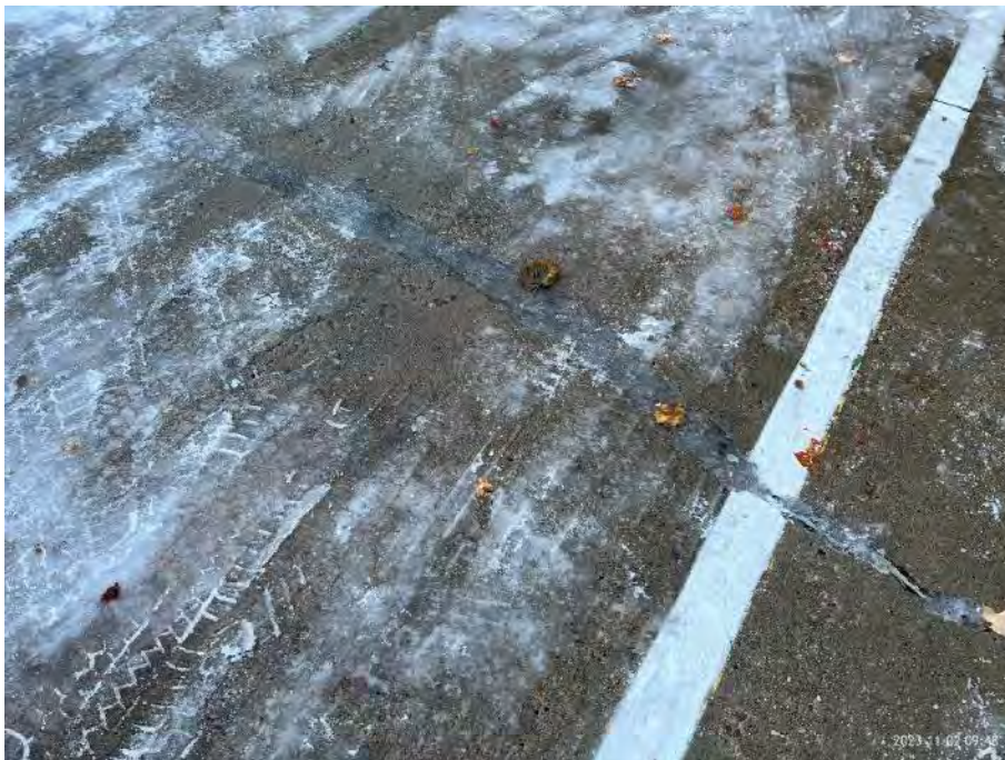
Photo 18 – Typical condition of wear slab concrete on garage was distressed.
