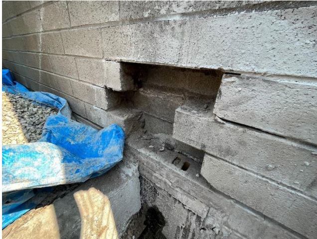
Figure 9: Destructive Test Opening 2 Overall. Note no thru-wall flashing.
