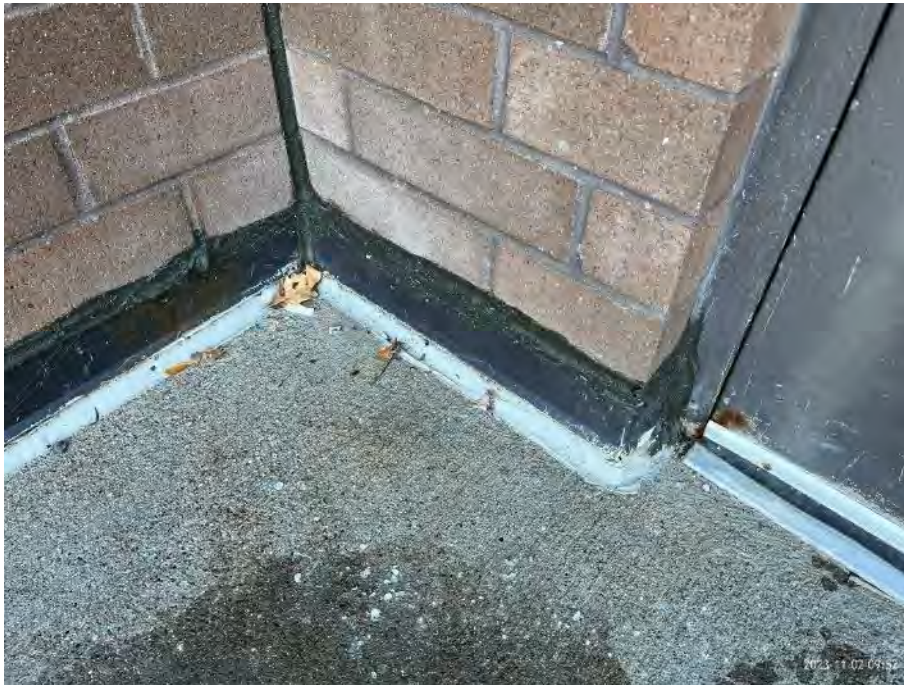
Photo 5 – Closer view at corner, east of service door, with thick bead of dark gray sealant at base joint of brick and no weeps visible.
