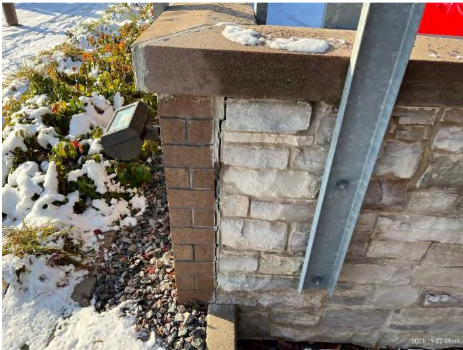
Photo 14 – North side of trellis wall corner at Grid C.9-22, large crack formed between brick and stone.
