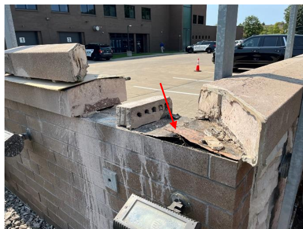
Figure 4: Existing flashing membrane under coping stone.
