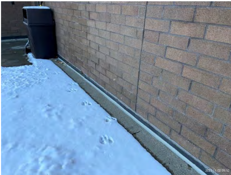
Photo 8 – West of service door, weeps still visible at base joint of brick,
