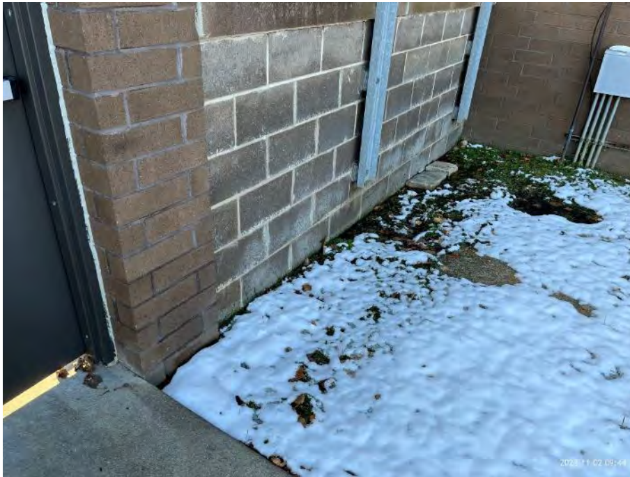
Photo 17 – West side of CMU trellis wall showing evidence of moisture.
