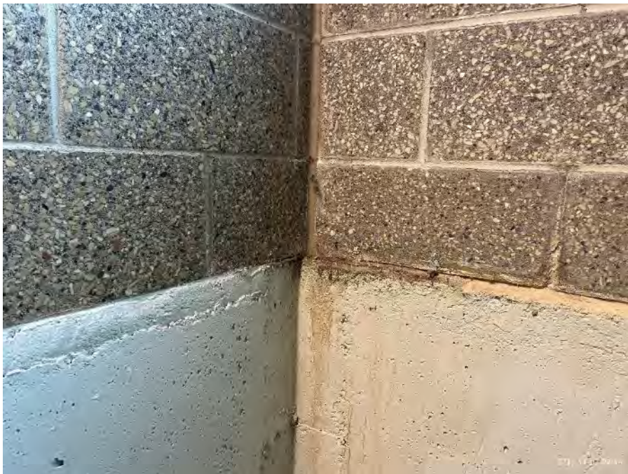
Photo 10 – Interior of Stair 'E', northwest corner, water staining along base mortar joint and interior of concrete wall.
