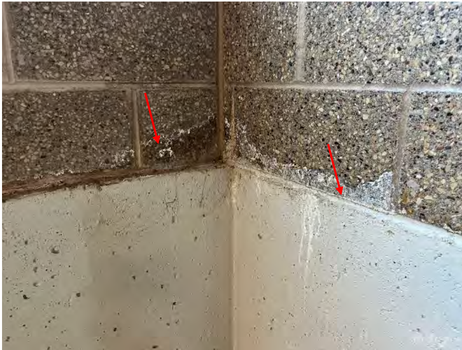
Photo 9 – Interior of Stair 'E', northeast corner, water intrusion, staining and efflorescence.
