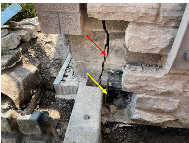
Figure 3: Crack in existing CMU wall (red arrow) and discontinuous waterproofing membrane (yellow arrow).
