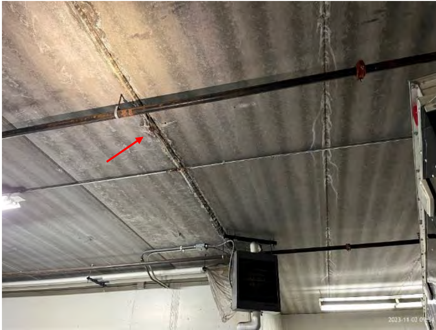
Photo 24 – View at plank joints looking north toward corner at C.9-22. Active leak at red arrow. Significant efflorescence at joints.
