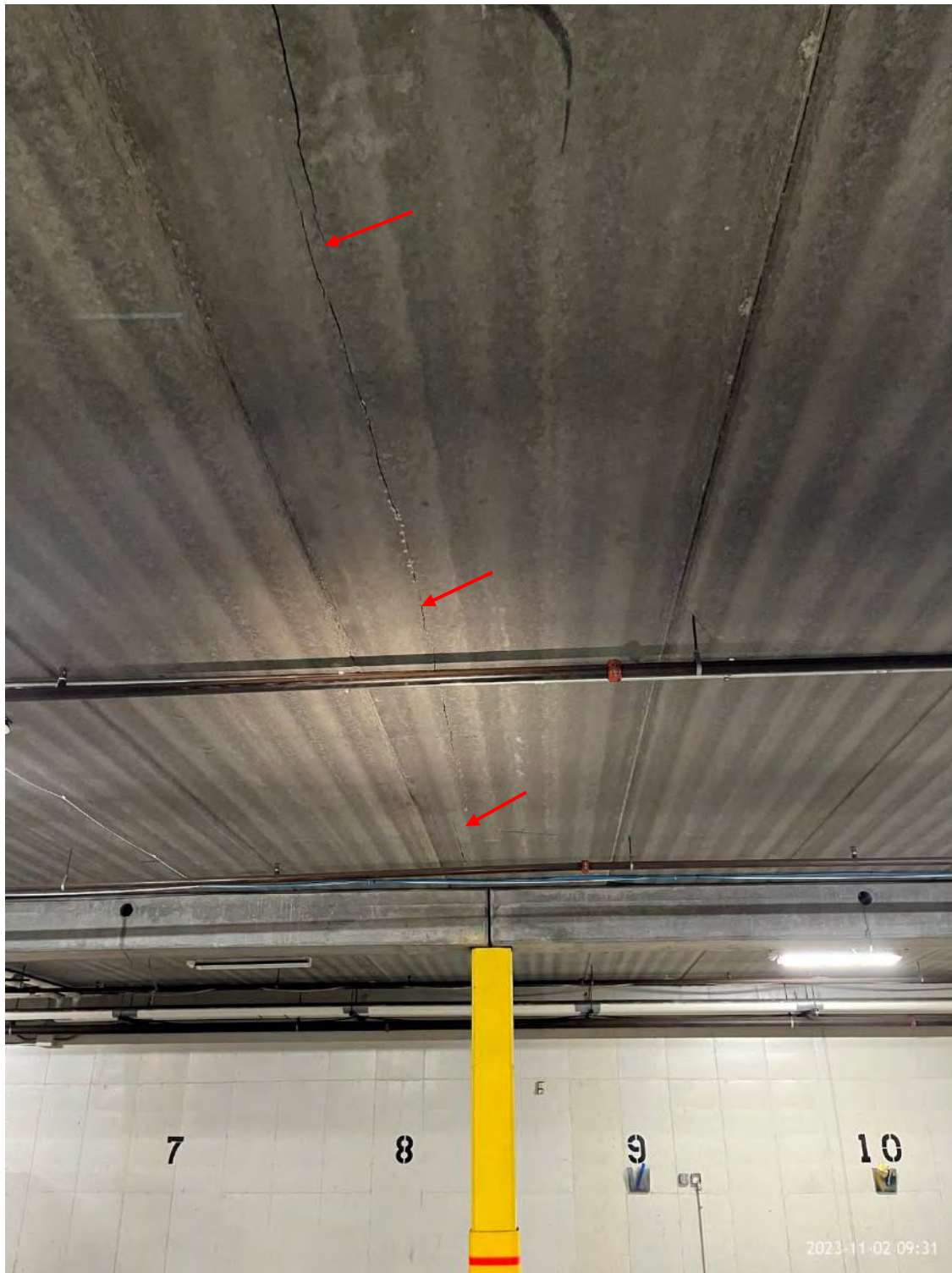
Photo 23 – Looking south along full-length crack along Grid C.9, under trellis wall. Minor efflorescence in crack.
