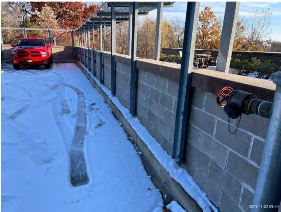
Photo 16 – West side of trellis wall, along Grid C.9, looking north. Some cracks at mortar joints and evidence of water intrusion.
