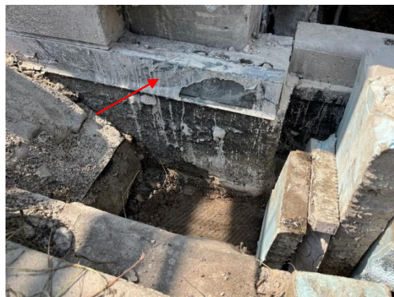
Figure 2: Plaza waterproofing up-turn at brick veneer with counterflashing. Note no thru-wall flashing.
