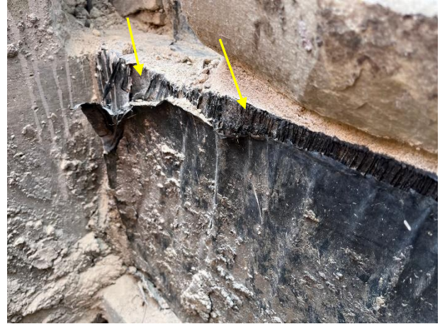
Figure 6: Deteriorated, unadhered and wrinkled below grade waterproofing.
