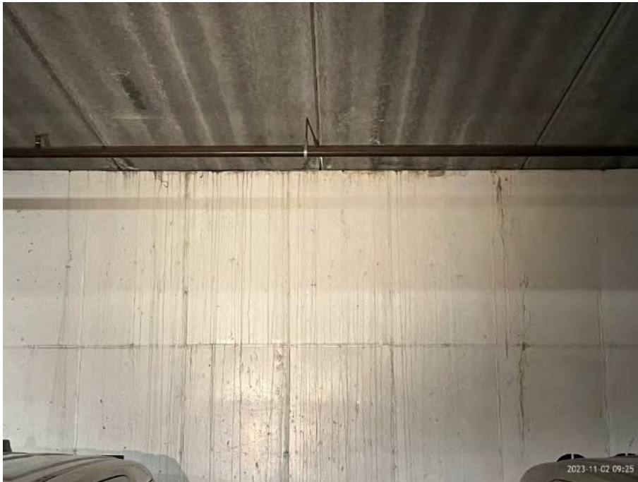
Photo 20 – Minor water staining along north foundation wall of garage.
