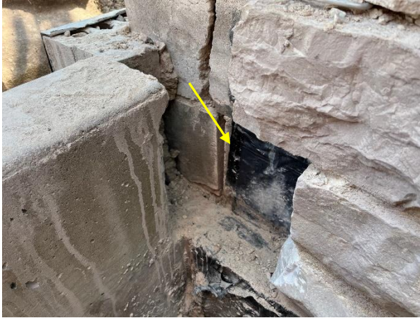
Figure 5: Discontinuous waterproofing at west side of concrete curb.
