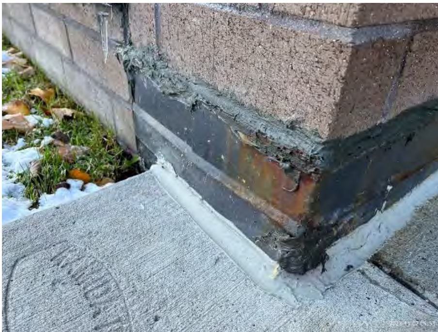
Photo 4 – Closer view at northwest corner of Stair 'E' exterior, with inadequately-tooled sealant applied at base joint of brick above metal flashing. Weeps covered by sealant or missing.
