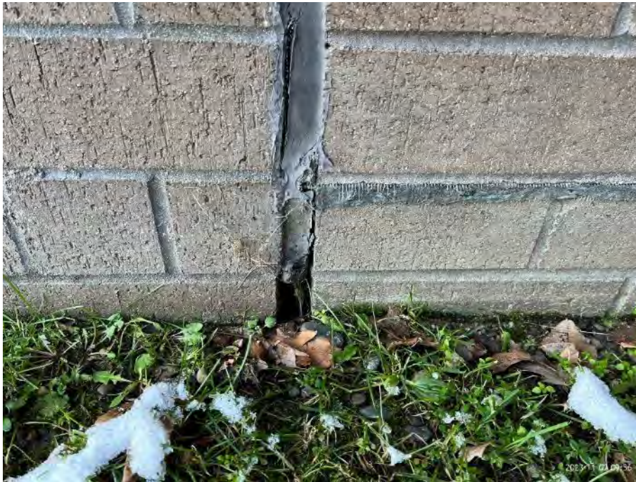
Photo 3 – Closer view at joint between original Public Safety Building and 2004 addition, missing joint sealant near grade.
