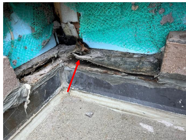
Figure 15: Unadhered through wall flashing membrane.
